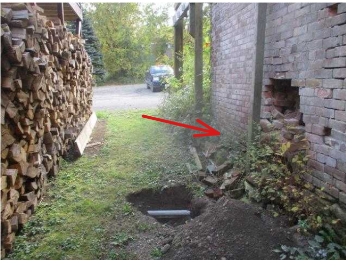
#5 main line comes in our building in the corner
