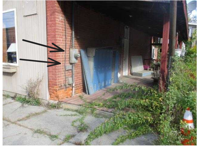
#14 Electric needs terminated but phone line needs to be diverted for fire department
