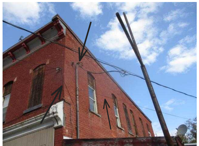
#12 phone line needs diverted for the fire department
