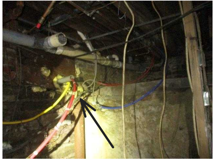
#34 Water lines that go to neighbor
