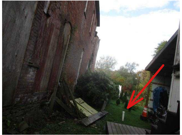
#4 Sanitary vent pipe
