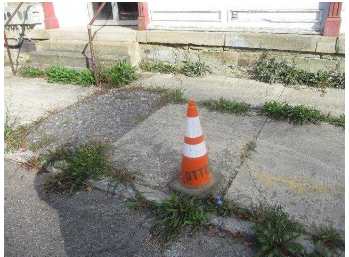
#16 Gas line already terminated
