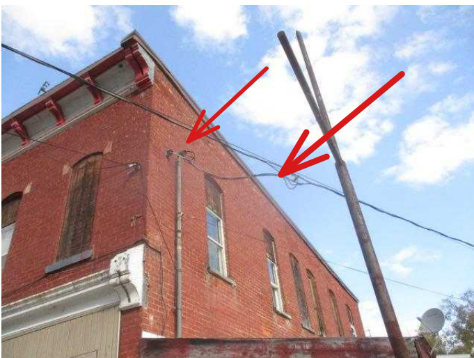
#11 Electric entrance cable on right side needs disconnected
